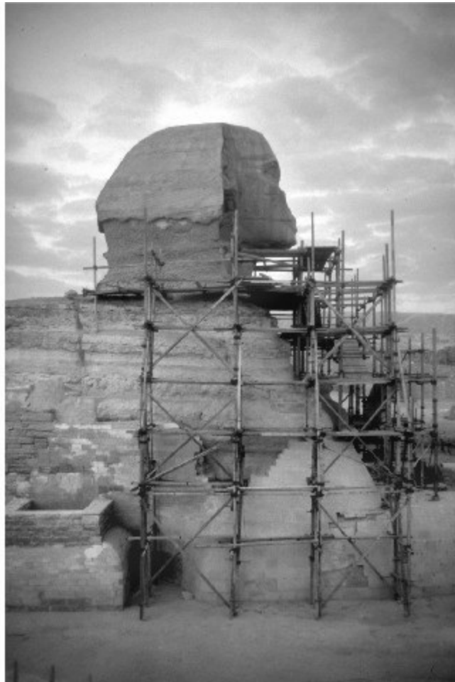
Fig. 11-6. Sphinx with flat headdress. Scaffolding shows that reconstruction and stabilization were taking place.
